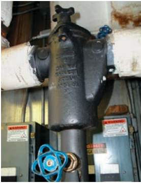
Inverted bucket steam traps are often used on larger air handling systems.
