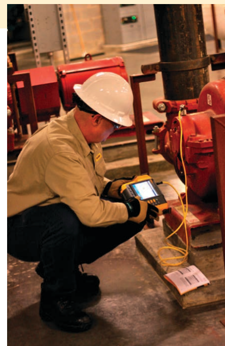
Many boiler plants distribute hot water to various building systems, and a vibration tester will indicate various pump problems and trend their severity over time.
