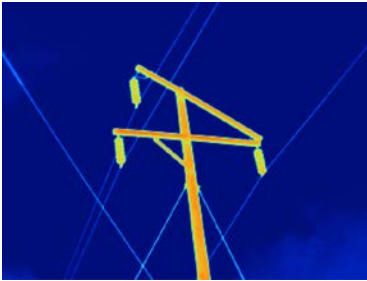
Figure 1: High voltage power pole, captured with a TiX560 camera and standard lens.
