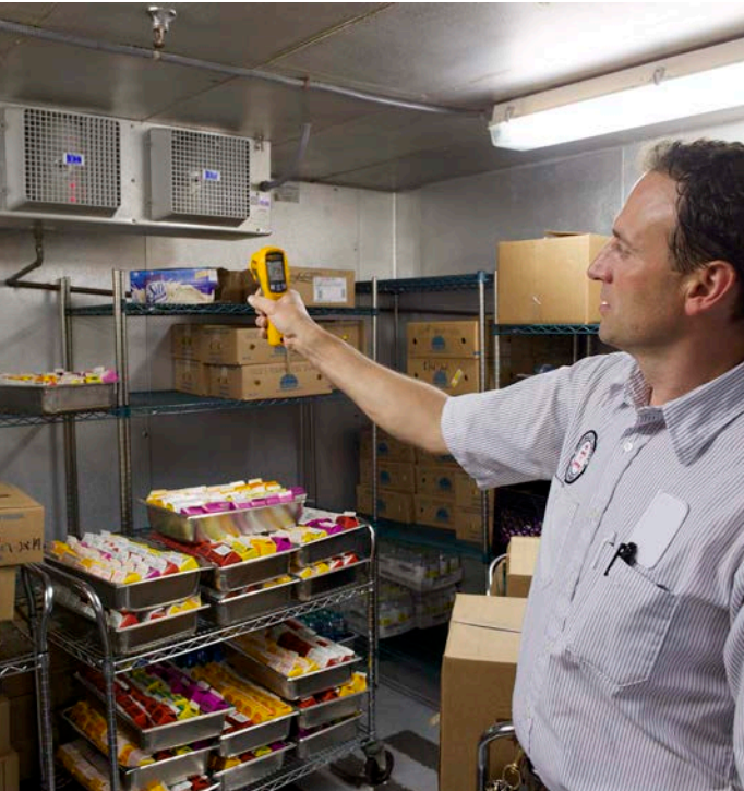
Mark uses his 62 MAX thermal imager to check refrigeration units in a walk-in cooler, as part of his preventive maintenance program.
