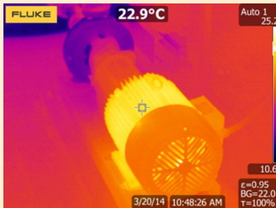
Combo: This heat pattern indicates an operational motor.
