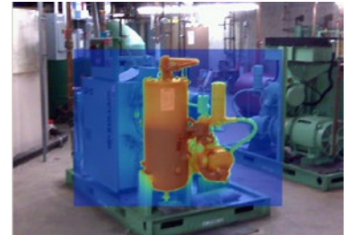
Industrial compressor, blending
