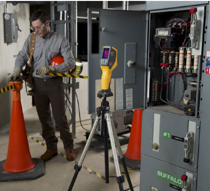
Automated monitoring alarms available on the VT04.
