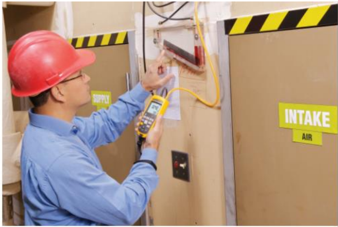
Figure 1: Checking pressure drop across the air filter with Fluke 922 Airflow Meter/ Micro-manometer
