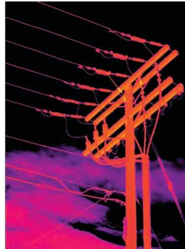
Electrical utilities broken strand and high resistance.
